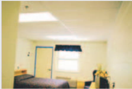
The new Polk Center includes accommodations for 24 people. Celotex Brand Baroque panels were used because they produce less reverberation and a higher degree of sound attenuation.
